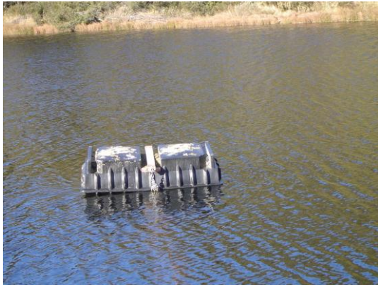
Pump intakes are not always what you would expect them to be.
